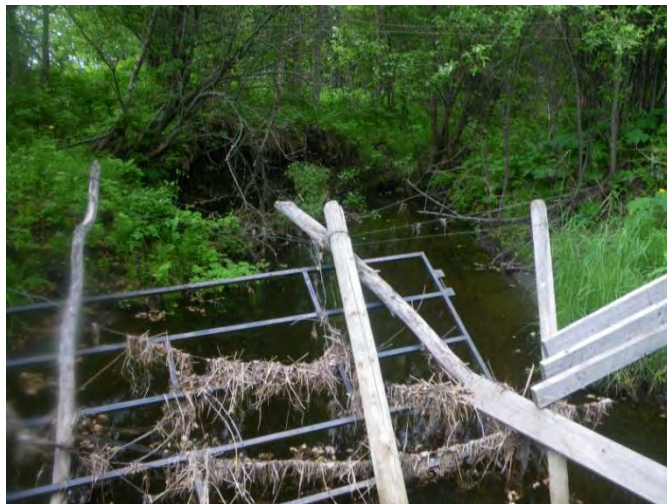
View upstream through the centre of the proposed pipeline corridor at 50 m downstream (19-06-14).
