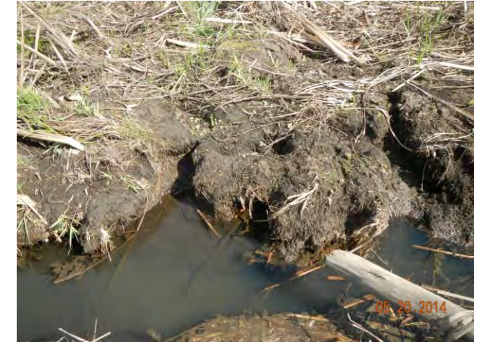
View of right bank approach at centre of the proposed pipeline corridor (20-05-14).
